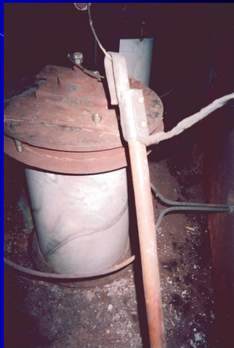
Cracked Support insulator
